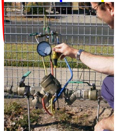
Setting up Test 1 on a Febco DCV
