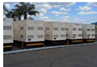
LOAD SHARING GENERATORS
